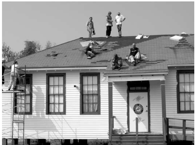
Plenty volunteers Neal Bloomfield, Joel Kachinsky, Jeffrey Keating, Jeffrey Clark and Carl Evertson joined with other volunteers to repair the roof of the Houma Tribal Office Building In Golden Meadow, LA.
